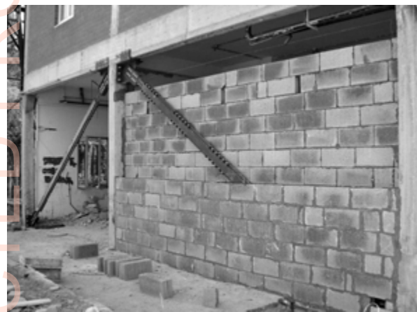
Figure 2: Top - Damage in the full scale building after the test on the original structure; Middle - First repair intervention, by means of FRP bars; Bottom - second repair intervention, by means of BRBs.
