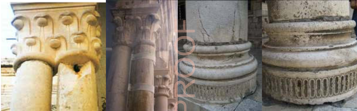
Figure 1: Fractures of column elements.
