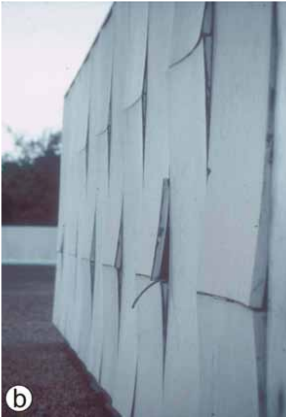
Figure 1: (a) Finlandia City Hall in Helsinki with deformed panels made from marbles, (b) Details of strongly deformed Façade cladding made of Carrara marble from Finlandia Hall in Helsinki.
