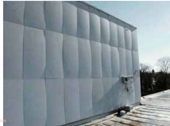
Figure 2: Lower Saxony State and University Library (SUB) showing a pronounced bowing of marble panels.
