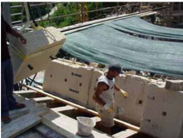
Figures 4&5: Axonometric view of the load bearing arch during the assembling stage, General Engineering WorkGroup (above), with a detail of construction (below).
